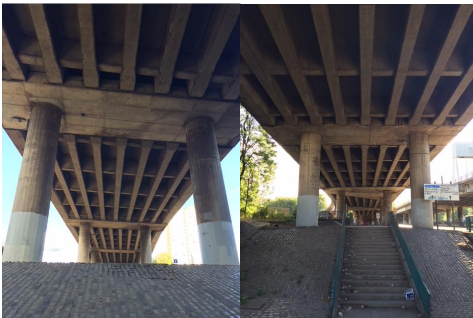
Figure 33: Underneath the M8 - Large concrete structures and litter.
