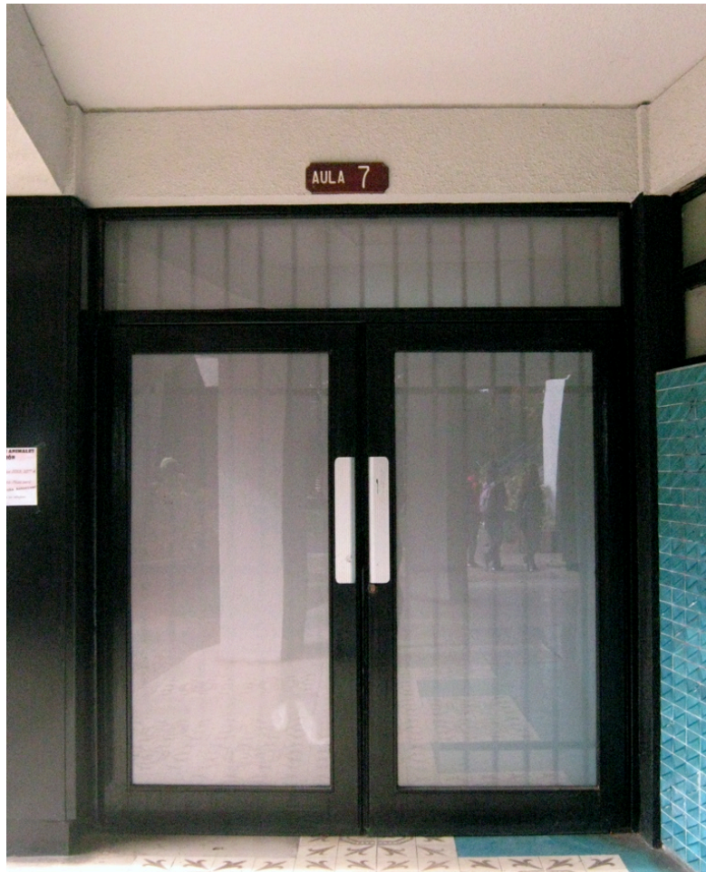
Figure 16. The door of the storeroom is a pull/push type of door, which is easily open when not locked with a key, and is not hermetic.
